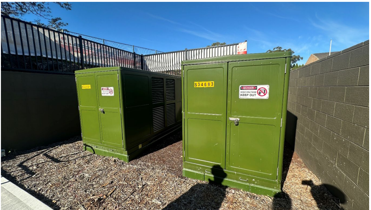
8. Completed substation near the Gate 2 (or H2) entrance. 23/06/2026
