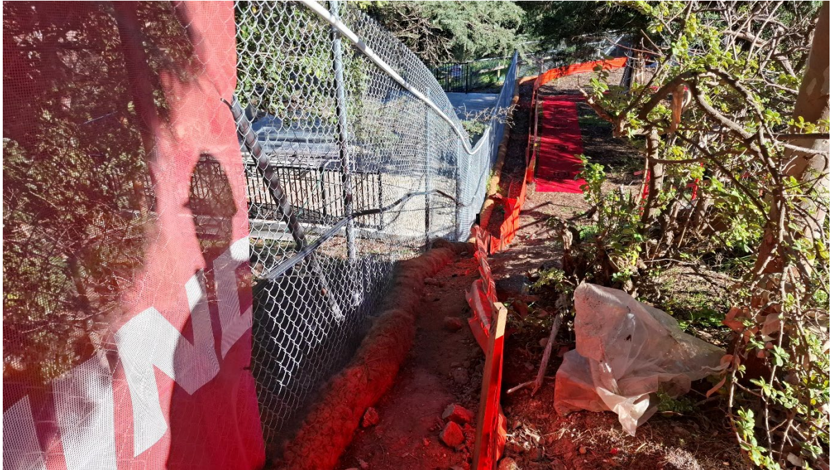
15. Implemented erosion and sediment control measures near the former pool. 23/06/2026
