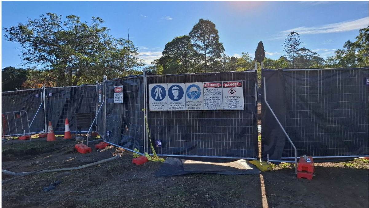
25. Asbestos warning signs around an area awaiting asbestos clearances. 23/06/2026
