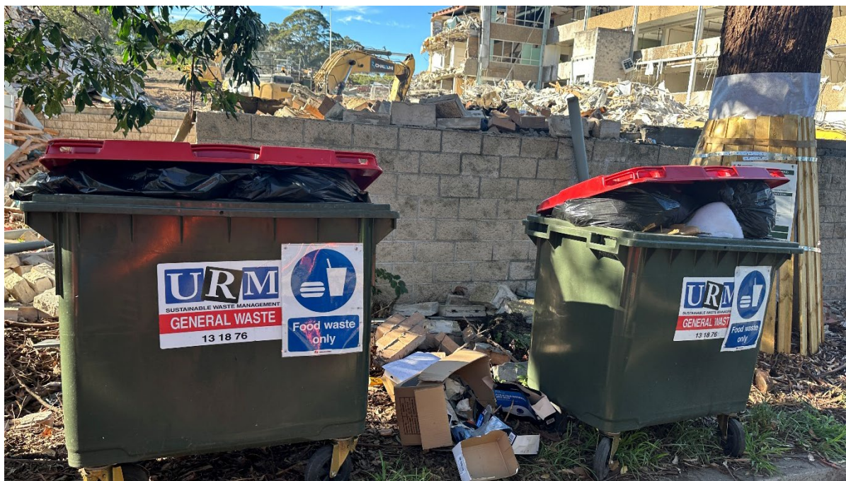
24. Portable waste skip bins located near the Gate 1 (H1) entrance ready for collection with some waste spillage. 01/05/2026
