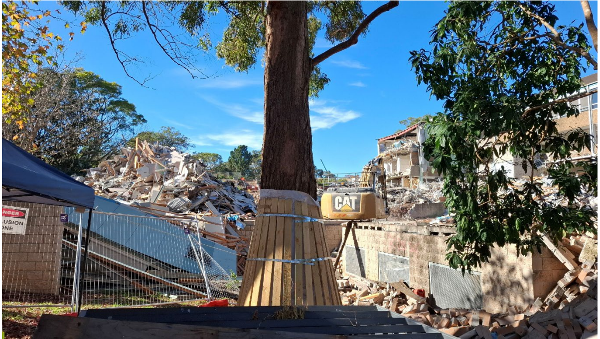
17. Implemented tree protection measures near the active demolition work zone. Part of the fence was damaged and in need of maintenance. 23/06/2026
