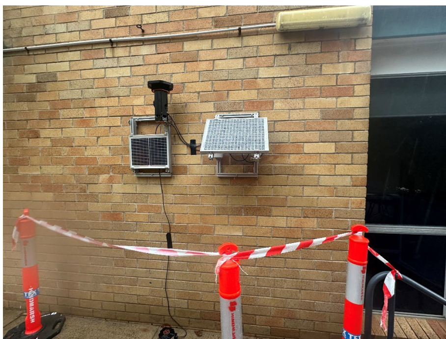
Photo 8: Hive monitoring system located to the south of the substation works area.
