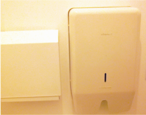
These paper towel dispensers cannot be seen against the wall by anyone with a sight impairment.
